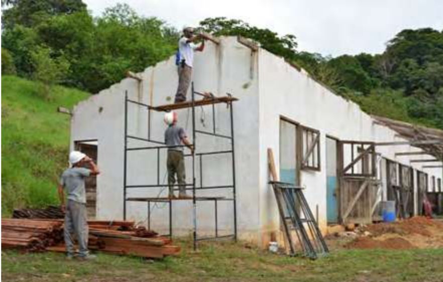
Refurbishment of the old horse stall that will house the cultural center.
